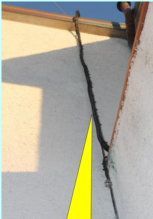
Cavi coax esterni
